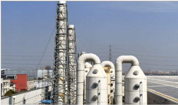
Exhaust Gas Treatment Facilities
