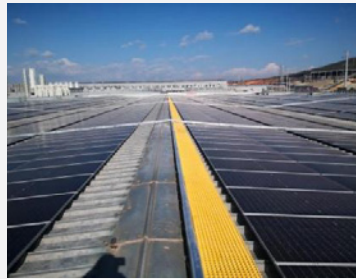
Rooftop Photovoltaic System at Yuhuan Base in Zhejiang Province
