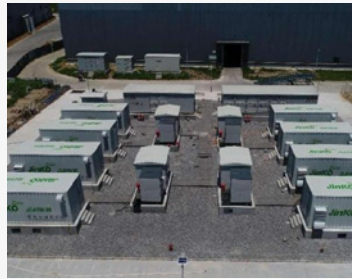
Energy Storage System in the Plant
