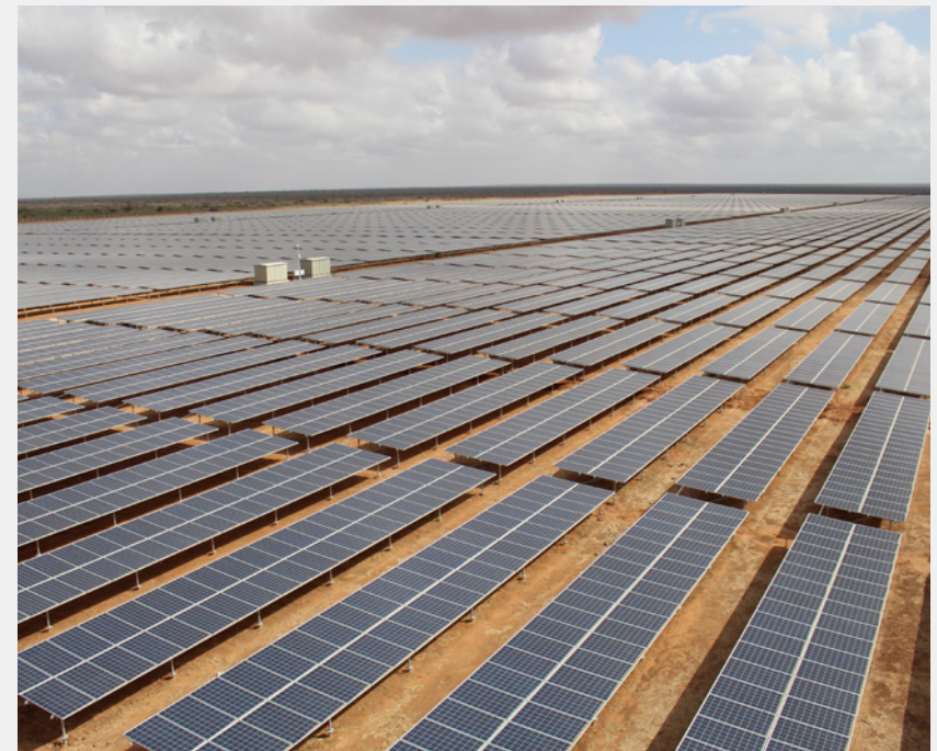
Garissa Solar Power Plant, the Largest Grid-connected Solar Power Plant in East Africa
